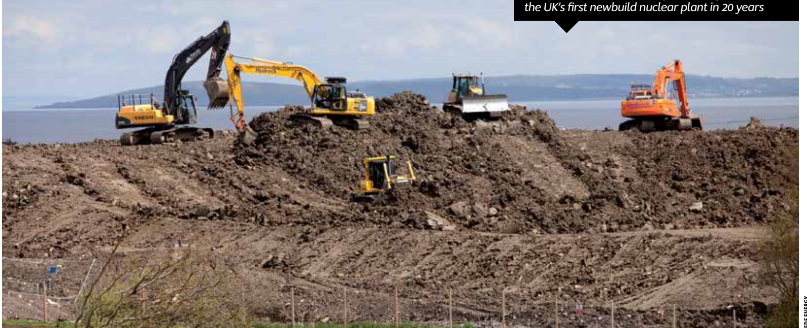
Groundworks are under way at Hinkley Point C - the UK's first newbuild nuclear plant in 20 years
